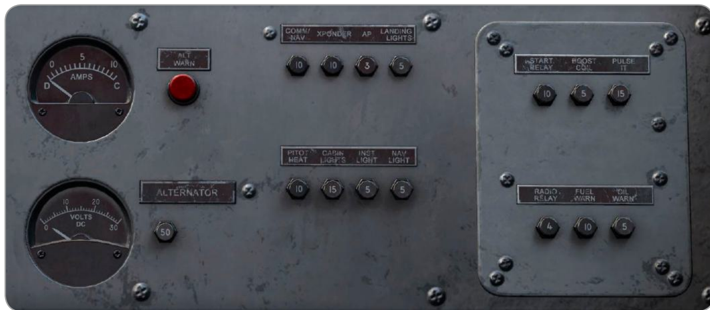
FIGURE 3-7 - ELECTRICAL SYSTEM INDICATORS & CIRCUIT BREAKER PANEL
