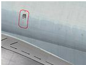
No Second Emergency Exits
