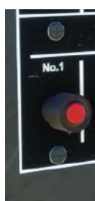
OFF OR TRIPPED / pulled in red
