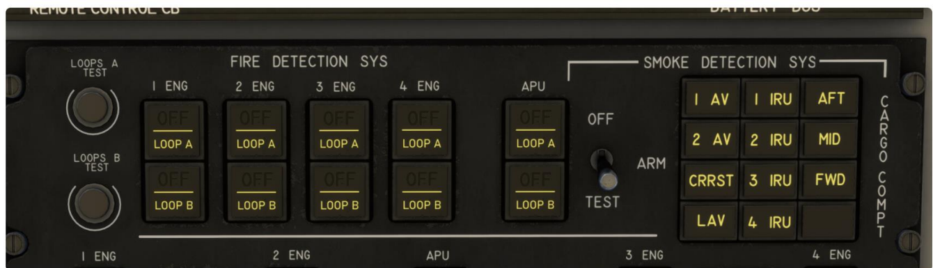
Fire Detection System
